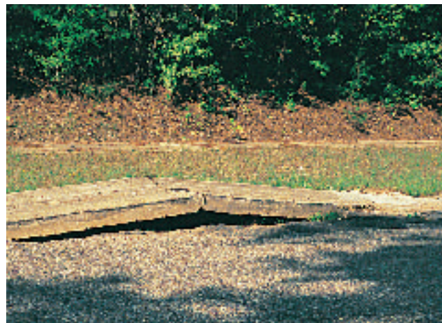
Figure 2 Most objects expand as their temperatures increase. Pieces of this concrete sidewalk forced each other upward when the concrete expanded on a hot day.
